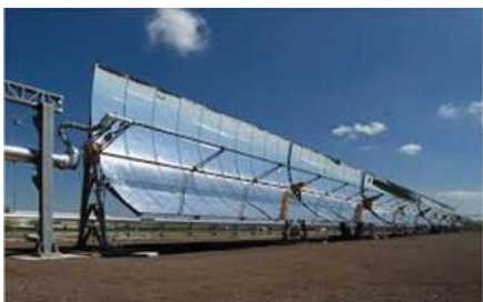
Demo plant of molten salt parabolic trough by Archimede Solar
