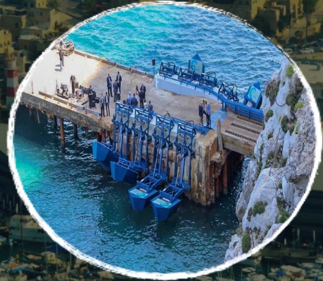
100 KW Power Plant
